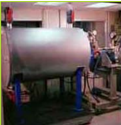
Biodigester In Mechanical Room
