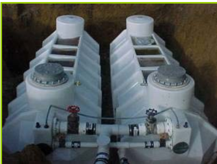
Dual Chamber Biodigester
