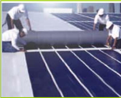
Thin-film BIPV roof system
