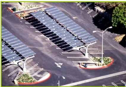
PV sun shades in parking lot
