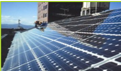
Monocrystalline PV sloped roof system
