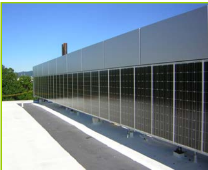
Polycrystalline PV Array used as an equipment screen
