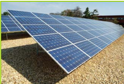
Monocrystalline PV Array mounted at a fixed angle to optimize output
