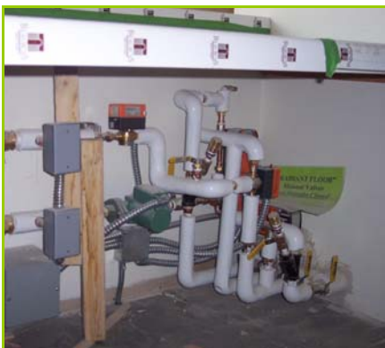
Manifold installation undercounter
