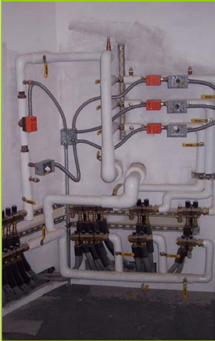
Manifold installation in janitor closet
