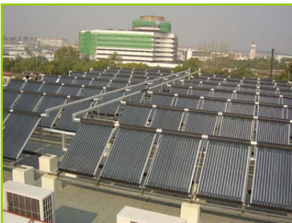
Evacuated Tube Collectors
