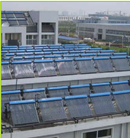
Evacuated Tube Collectors
